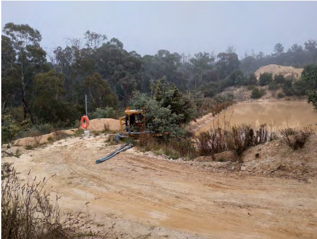
Plate 17 Pumping infrastructure in place adjacent southern sediment dam
