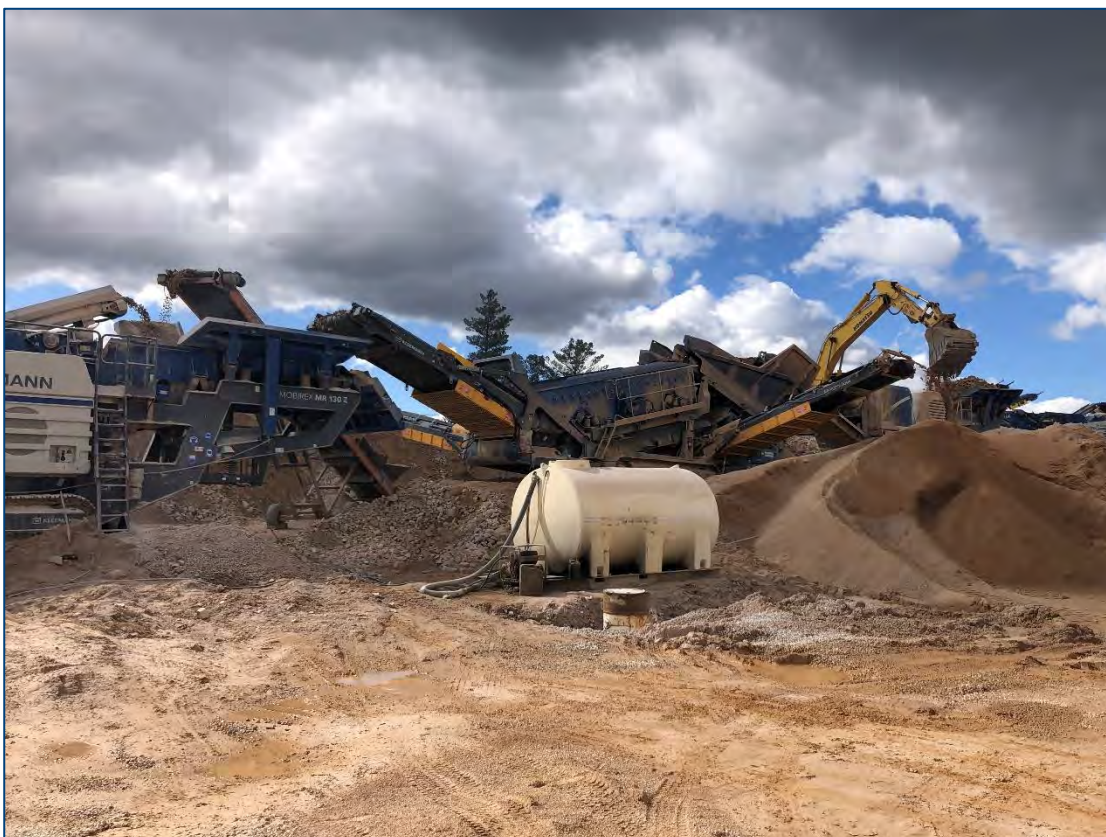
Photo 4.5 Aggregate Crushing Train
