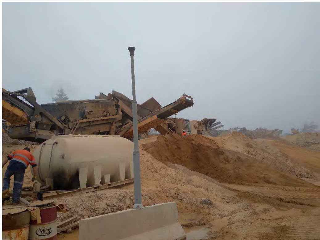
Plate 4 Process water tanks located at in-pit screening area
