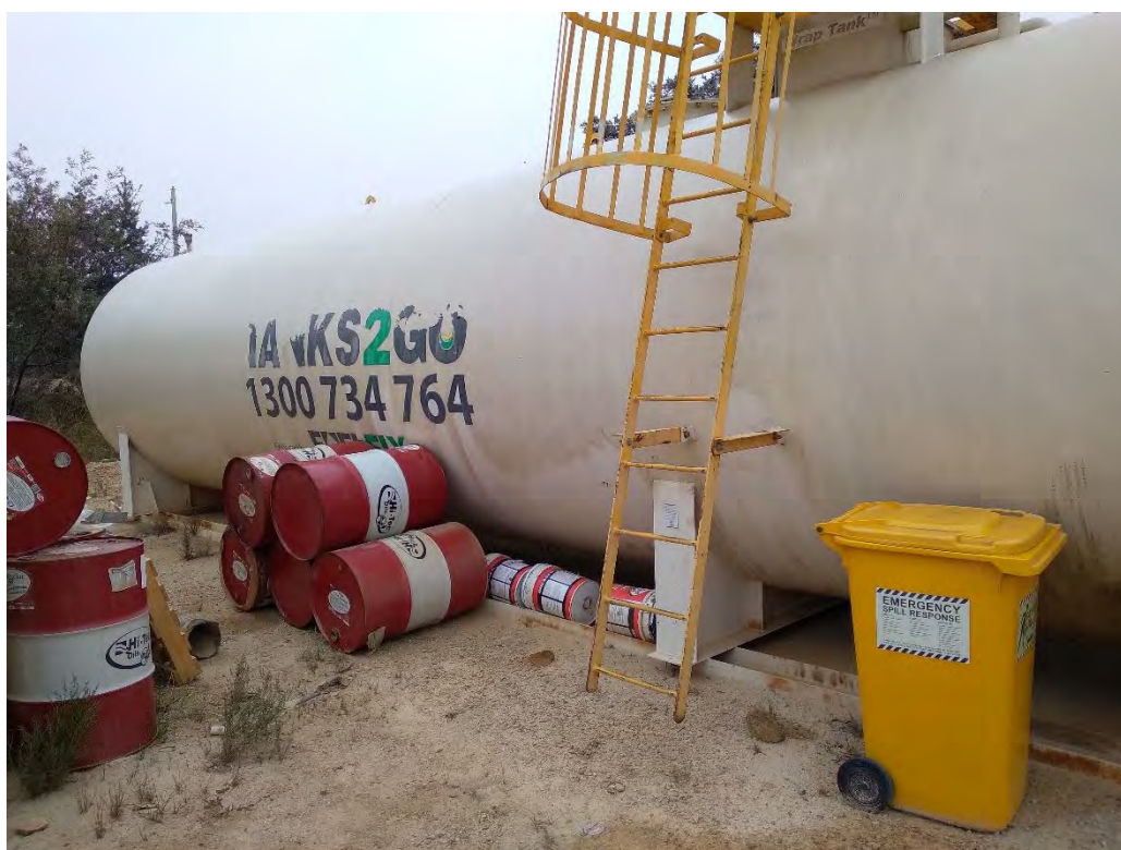
Plate 15 Bulk diesel storage tank and spill response kit
