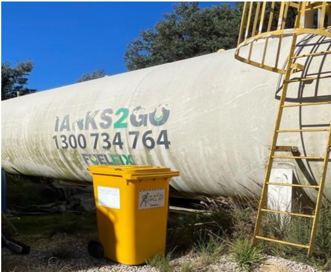
Plate 14 Onsite refuelling area and storage tank
